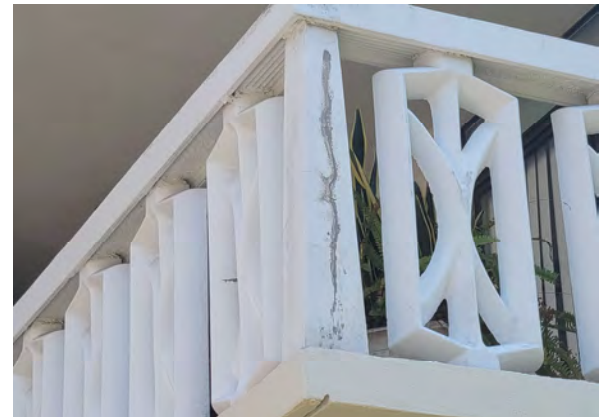
20 Support Column Crack
