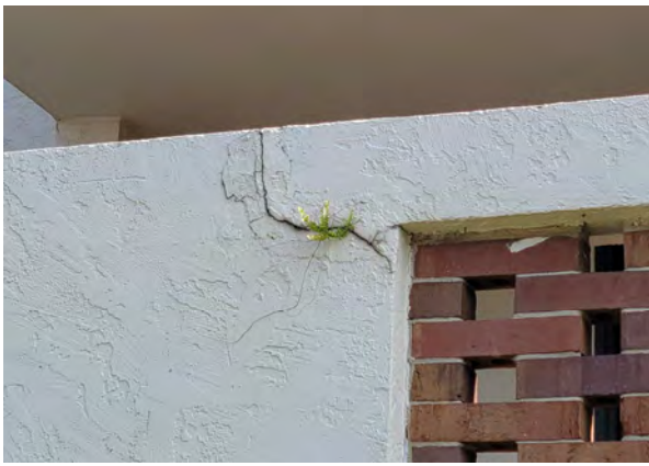
17 Cracks in Patio Wall
