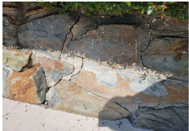
Retaining Wall Crack
