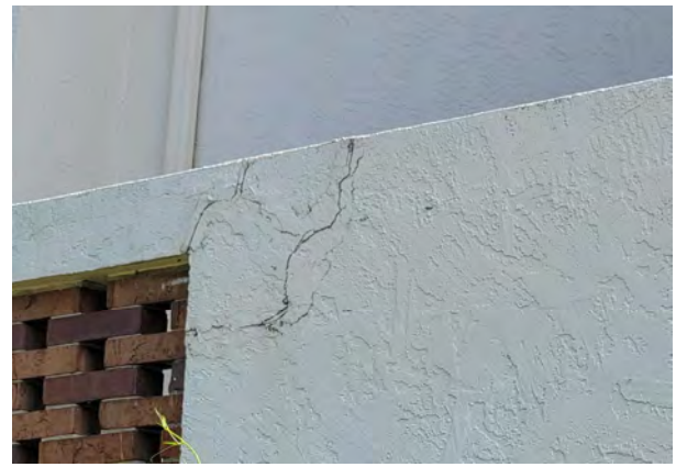
18 Cracks in Patio Wall
