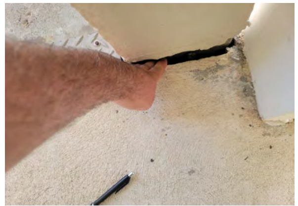
16 Gap at Column
