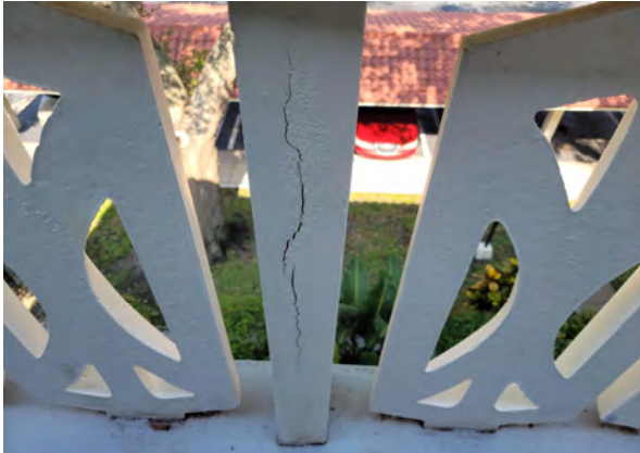
19 Support Column Crack
