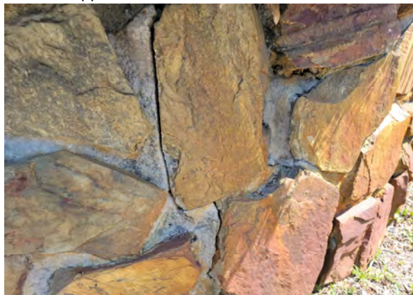
21 Retaining Wall Crack
