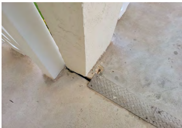
15 Gap at Column Overview
